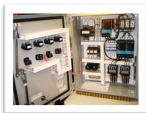
Clarifier Control Panel
