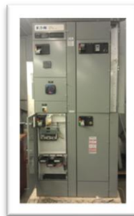
MCC and Power Panel
