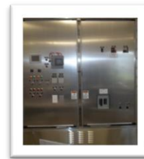
Triplex Pump Control
