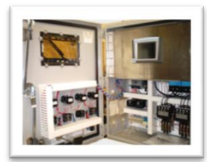
Simplex Pump Control
