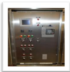
Duplex Pump Control
